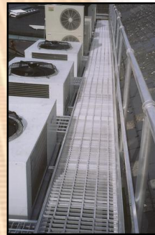
Alloy framed walkway fitted with open mesh alloy panels removable for gutter cleaning,
