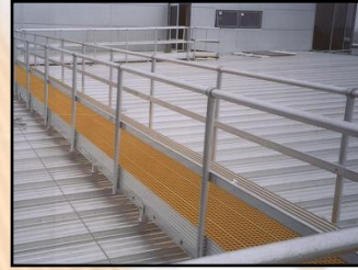
Alloy framed walkway with GRP decking fitted to standing seam roof panels.
